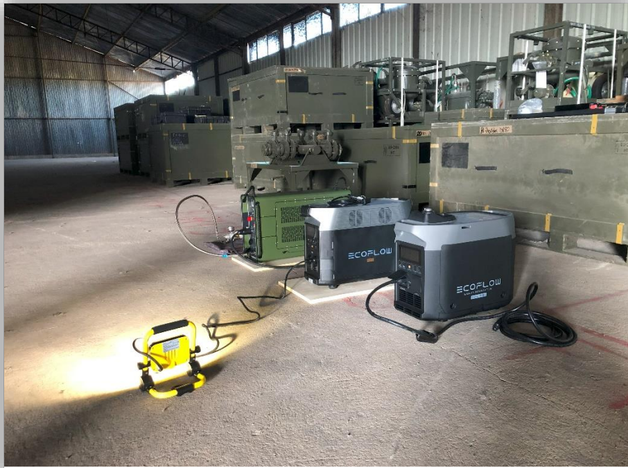
Figure 5: 1kW device connected to battery storage and GenSet (NATO ENSEC COE)
