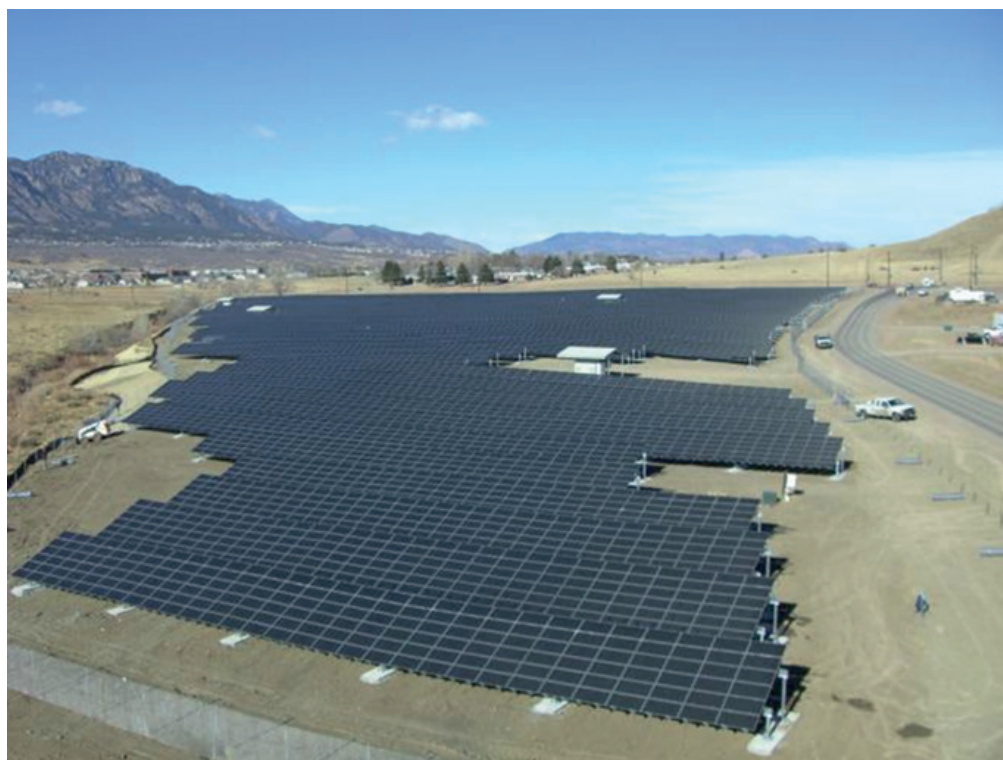
A two-megawatt solar array at Fort Carson, Colorado produces enough energy for 540 homes.
