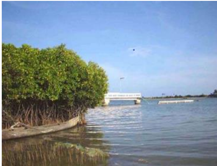
Figure 12: Boat jetty in the Vellar estuary (south-east coast of India) broken into pieces by a tsunami induced surge on the 26 th of December 2004 in the background. The foreground shows an artificially established intact mangrove forest (Kathiresan 2012).
