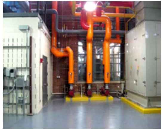
Figure 5 Central Utility Plant Micro-grid, Federal Research Centre, White Oak, Maryland
